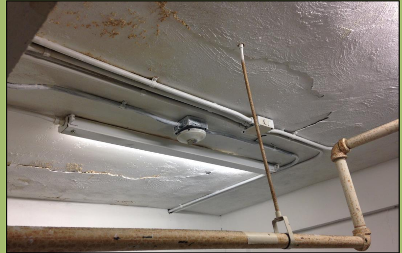
#2 Ceiling water damage 11/2015 Pre-rehabilitation
