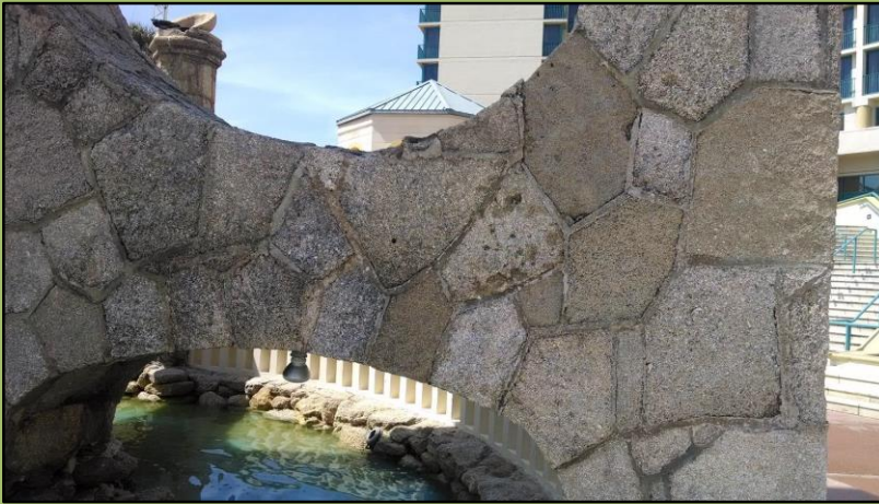
#1 Condition of coquina 5/27/14 Pre-rehabilitation
