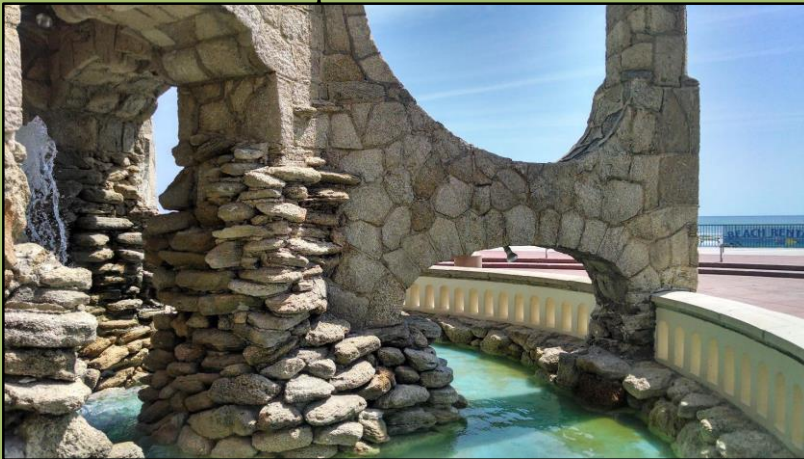
#2 Condition of coquina 5/27/14 Pre-rehabilitation
