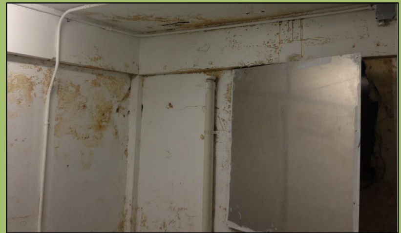
#3 Wall Condition 11/2015 Pre-rehabilitation
