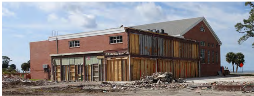
At severely-damaged buildings, repair work could cause unintended collapse.
