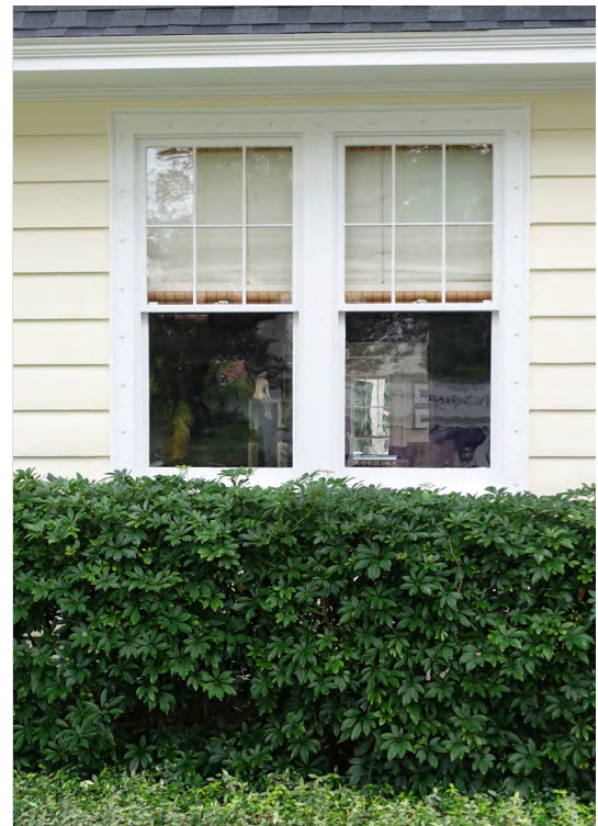
Historic windows are a character-defining feature and should be preserved if possible.
