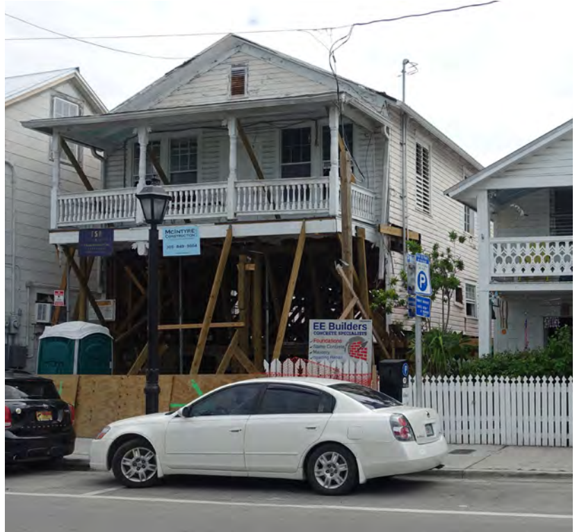
This building being elevated in Key West required a new foundation, making it exempt from the local definition of Substantial Improvement.
