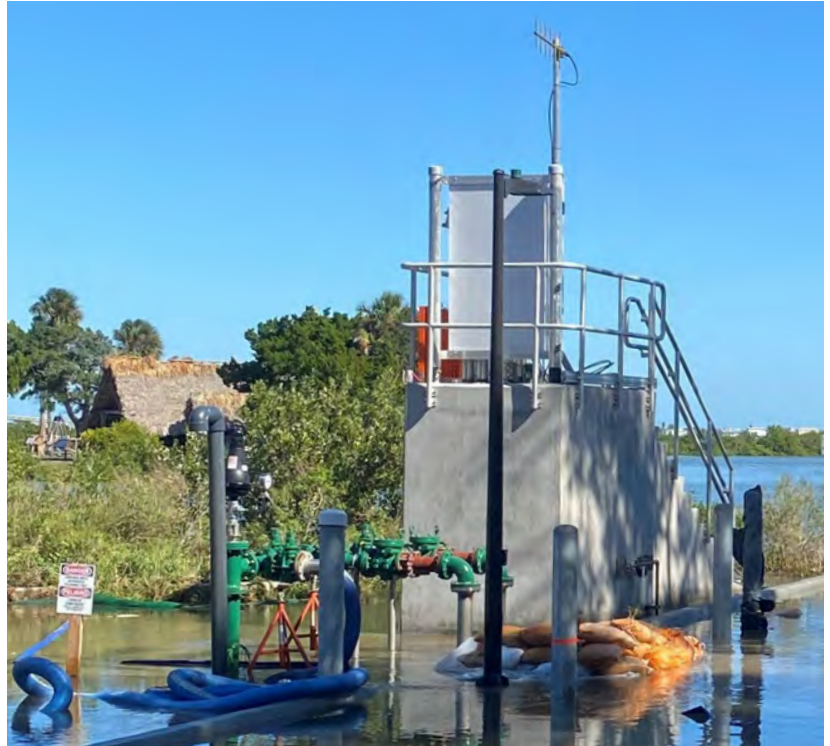
Pump stations elevated out of the floodplain provide the best chance of continued service during flooding and can impact natural views.
