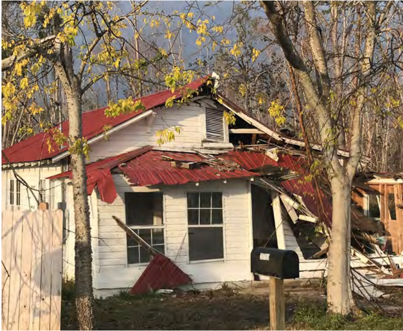
Historic properties that are deemed substantially damaged may need to meet additional code requirements during the repair process.
