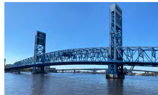
Bridges are a part of local and state infrastructure that require a lot of maintenance investment.
