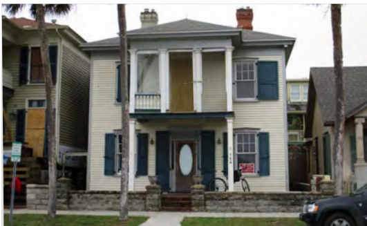
The condition of a building may impact the ability of the structure to be elevated.
