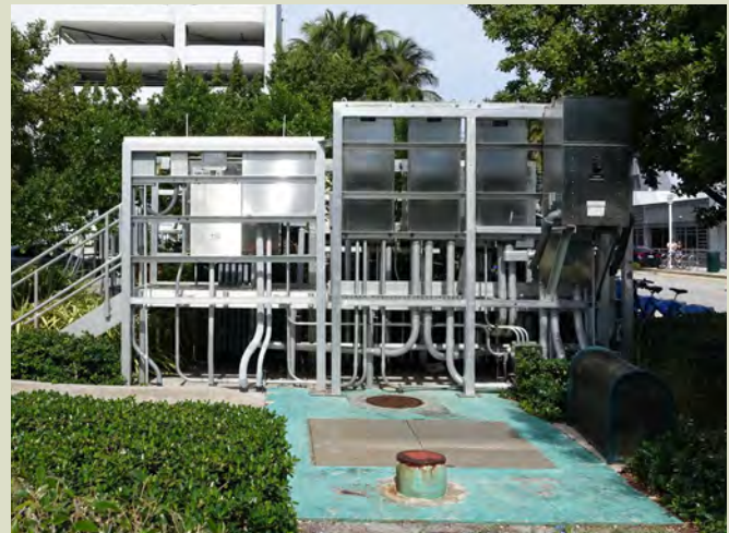
Massive pump stations in Miami Beach constructed above the floodplain to mechanically control stormwater flow.
