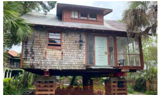
Elevating a historic building to a new foundation height can alter the individual building and the surrounding historic streetscape.
