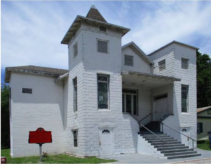
Lightning struck one of the identical roof towers of this historic church and fortunately the impact was limited and only affected the right tower roof.
