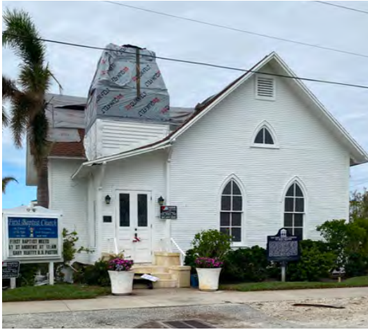
The First Baptist Church of Boca Grande experienced wind damage to the roof and steeple from Hurricane Ian in 2022.
