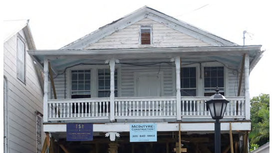
Building elevation projects can create a long period of time that the home is unoccupied and risk losing homestead exemption status.
