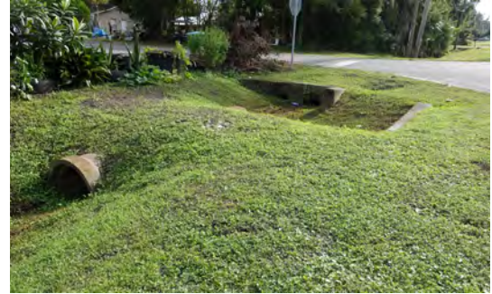
Concrete pipes under roadways connect culverts to serve as a drainage ditch.
