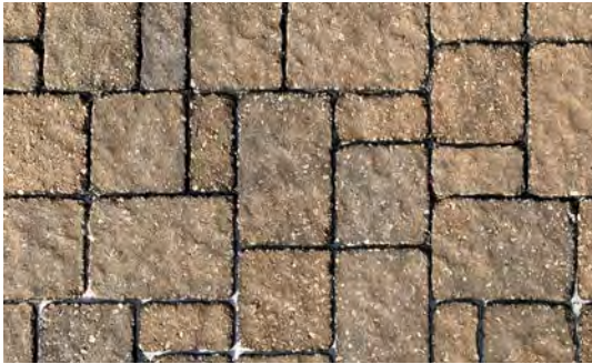
The spaces between pavers can absorb stormwater, but regular cleaning is required.
