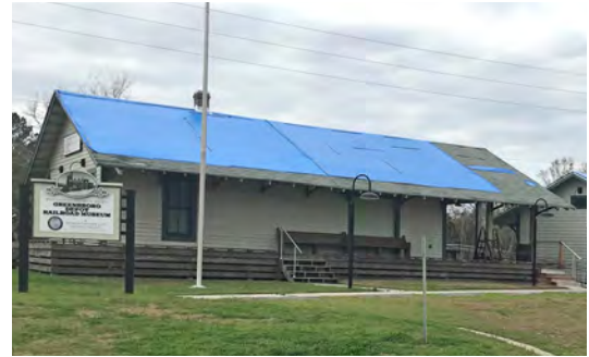
Wind damage from Hurricane Michael reached northward of Tallahassee into many rural communities like Greensboro.
