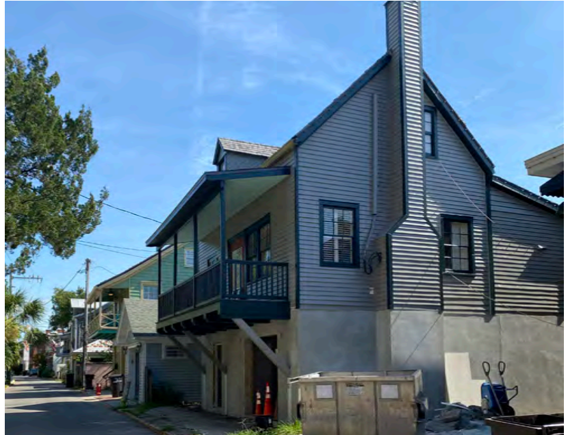
A building was elevated and garage space was added to the ground floor.
