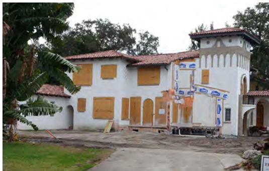
Substantial Improvement requirements can require other changes to meet the building code.
