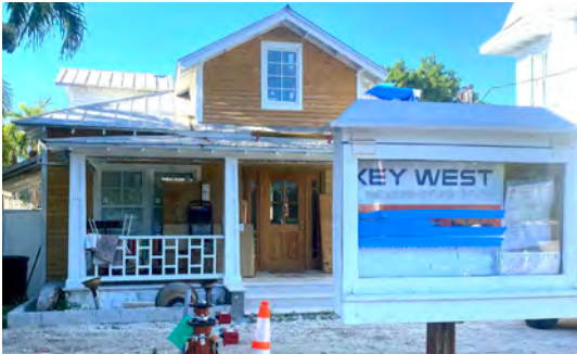
Historic properties are afforded some flexibility in the Florida Building Code for flood mitigation.
