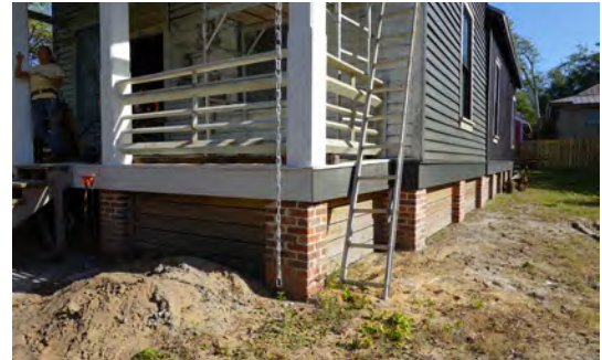
A historic building was elevated and constructed with a new brick pier foundation compatible with the original building.
