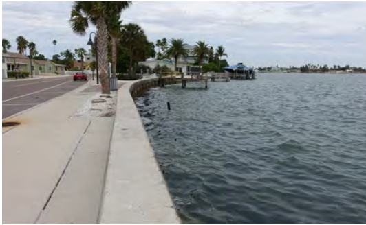
Seawalls such as the one in St. Pete Beach require maintenance to provide the best protection.
