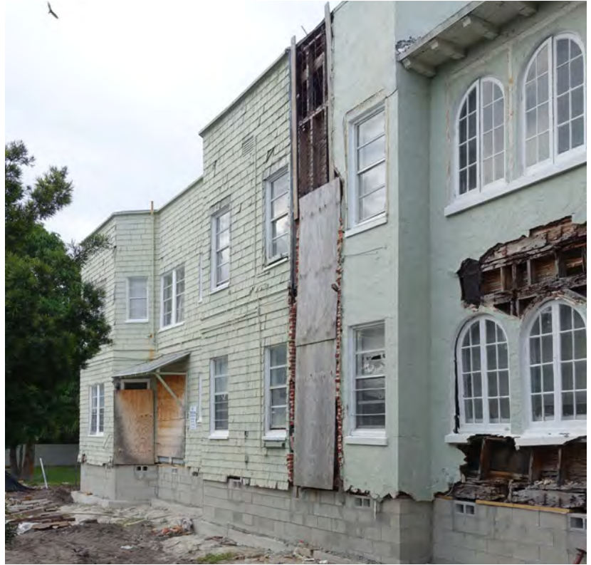
A large renovation exposing the structure is an opportunity to implement an Advanced Mitigation Package.
