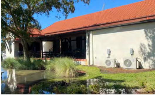
Mechanical systems are vulnerable to flooding and are often required to be elevated.
