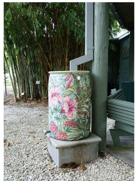
Stormwater can be collected in rain barrels and provide water for irrigation.
