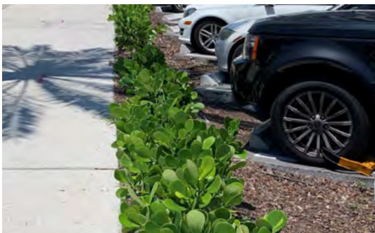
The asphalt has been removed from the edge of this parking area to provide a landscaped area that collects and absorbs stormwater runoff.
