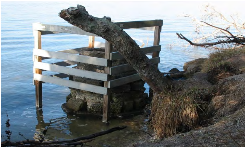
A colonial well been stabilized for preservation on site but is being lost to erosion.
